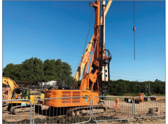
Installing our largest rotary bored piles at 1220mm at Wichelstowe for M4 underpass
